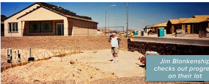
Walls in place helped potential buyers image where their homes would be
